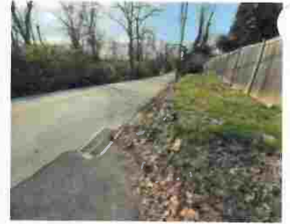
Roadside obstructions near Township Line Road, Whipton Township
